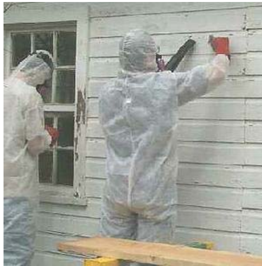
Workers remove lead-based paint from a home in Kansas City, Missouri. (Photo courtesy Project Lead Safe KC )
